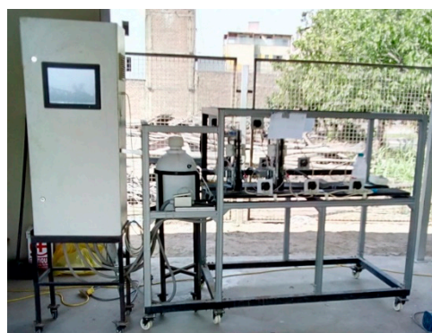
Figure 2. The ferrate(VI) reactor installed in the treatment plant.
